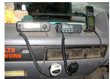
GRN and VHF radio installation
