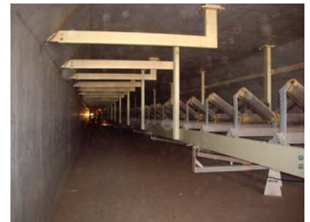
Coverage was provided to tunnels
