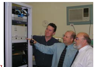
Teamtalk site equipment during factory acceptance testing
